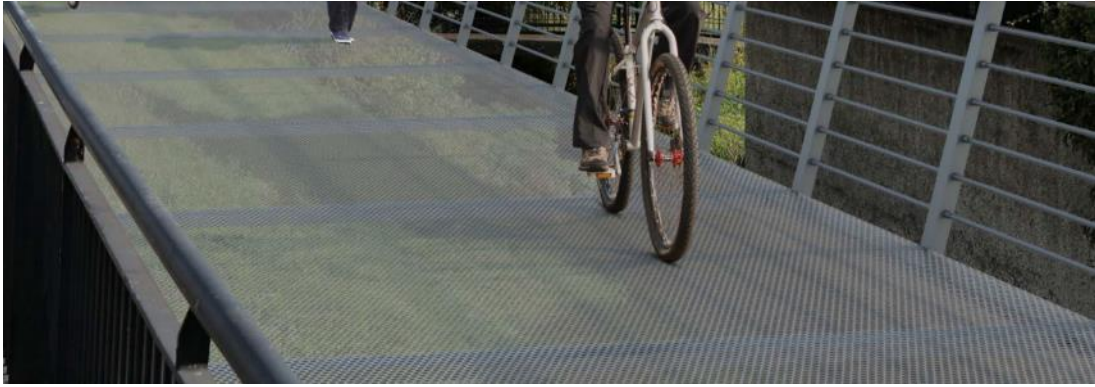
Figure 2-2-8: Close-up view of the proposed Stone Boat Boardwalk (EIAR Volume 3, Chapter 17, Figure 17.2.1.2)
